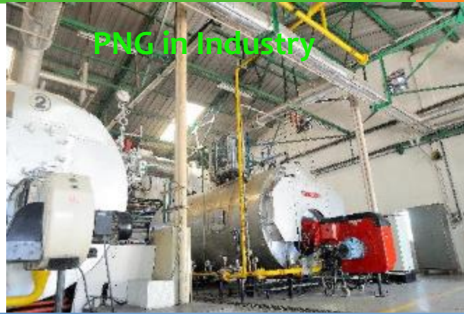
Natural Gas Skid
