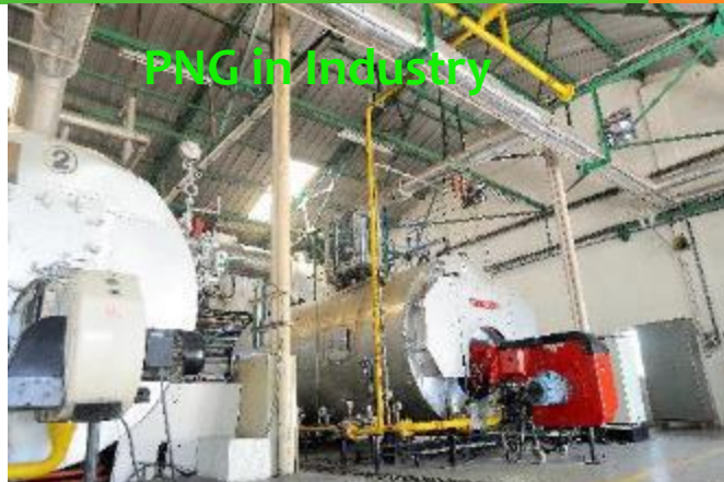
Natural Gas Skid
