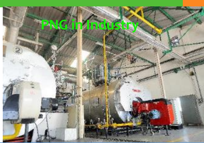
Natural Gas Skid
