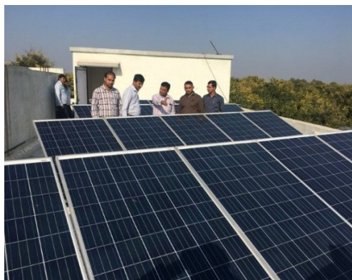
Solar panel at CNG station
